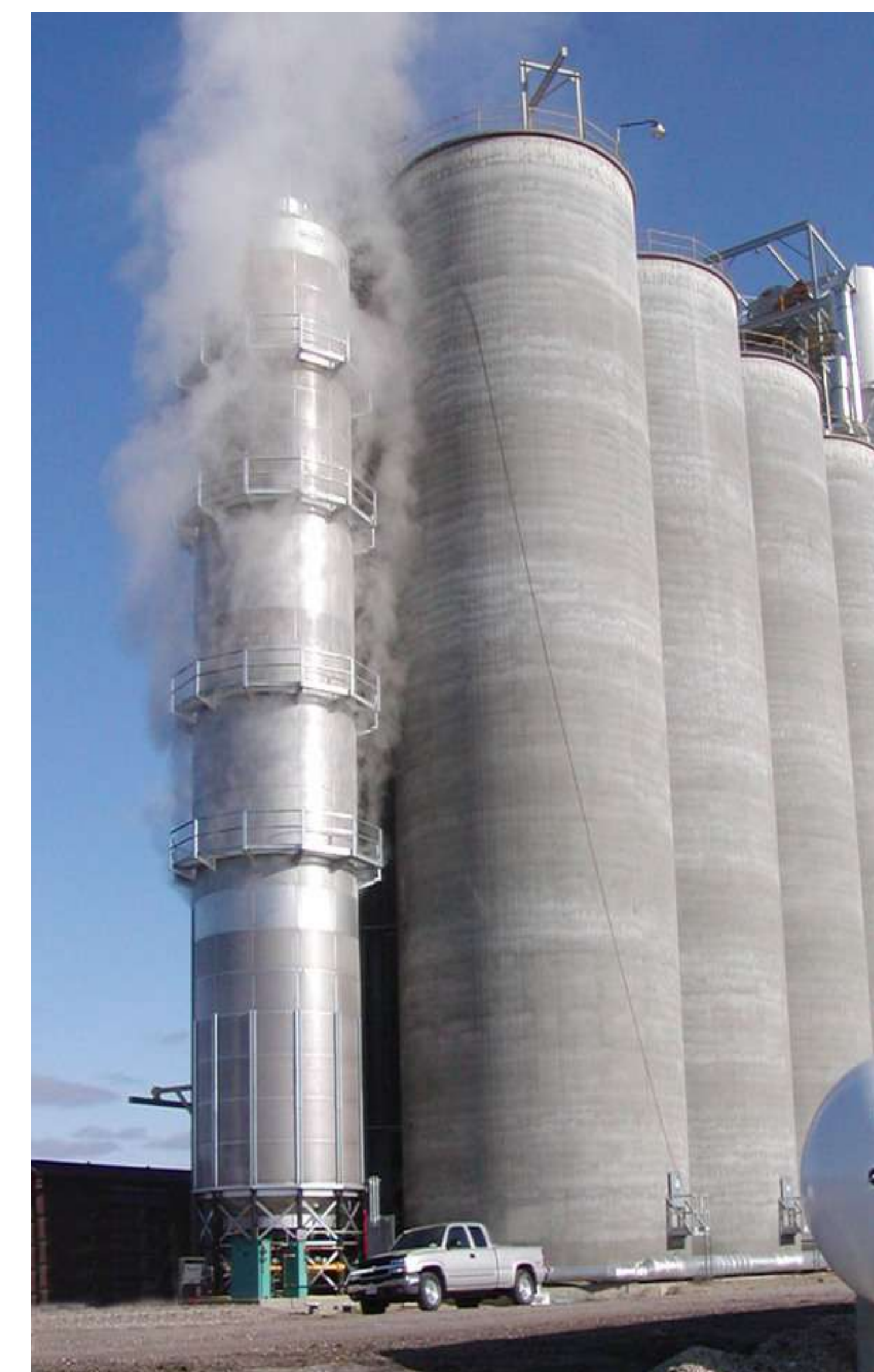
Typical tower dryer found at an ADM facility
